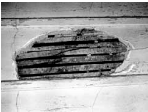
This beaded ceiling in one of the bedrooms of the 1847 Lockwood House, Harpers Ferry, West
