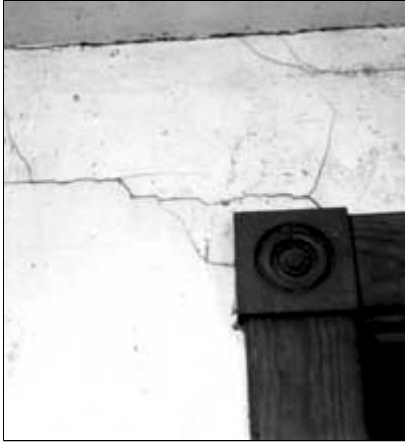
Stress cracks in plaster over a kitchen door frame can be repaired using fiberglass mesh tape and joint compound. Photo: NPS files.
