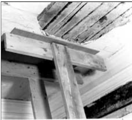
When ceiling repairs are made with wet plaster or with an injected adhesive mixture, the old loose plaster must be supported with a plywood brace until re-keying is complete. Photo: John Leeke.
